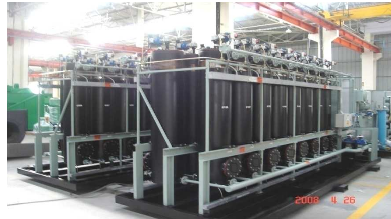
Transformer Oil Regeneration Plant
